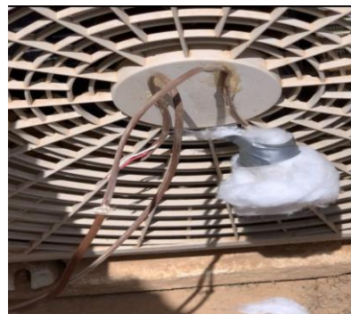
Figure 6 Installation of a thermocouple sensor for temperature measurement on the external air conditioning unit.
